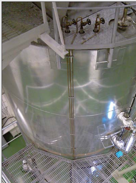
Marine Auxiliary Boiler
